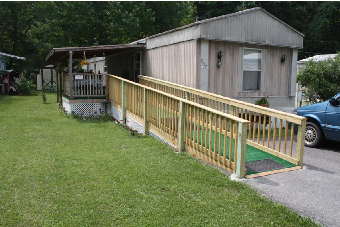
Figure 3 Alternate construction with decorative spindles. This ramp does not have the optional middle rail. The carpeting was added by the consumer and is not necessarily recommended by the NWVCIL.
