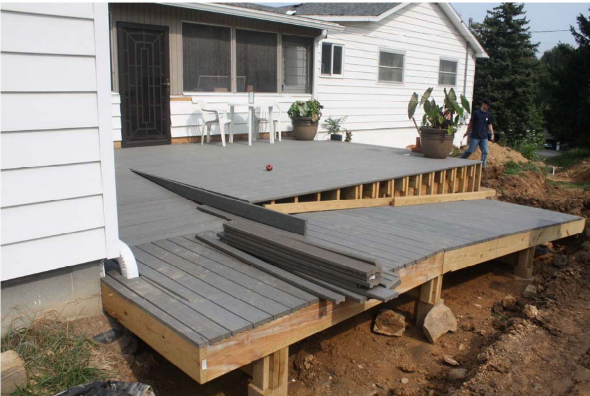
Figure 2 This ramp is unfinished, but notice the deck materials and density of support structure.
